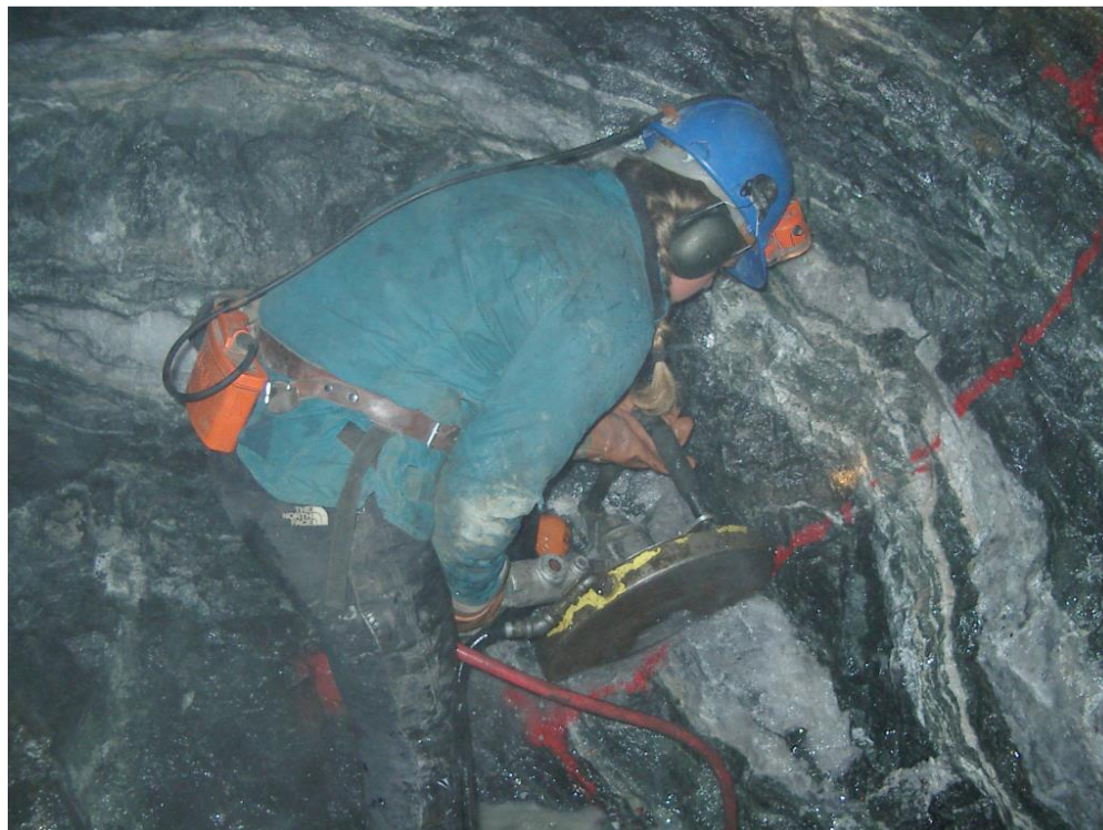
FIGURE 9.1 CUTTING A CHANNEL SAMPLE ON THE DEVELOPMENT FACE WITH A PNEUMATIC DIAMOND ROCK SAW AT BINGO
